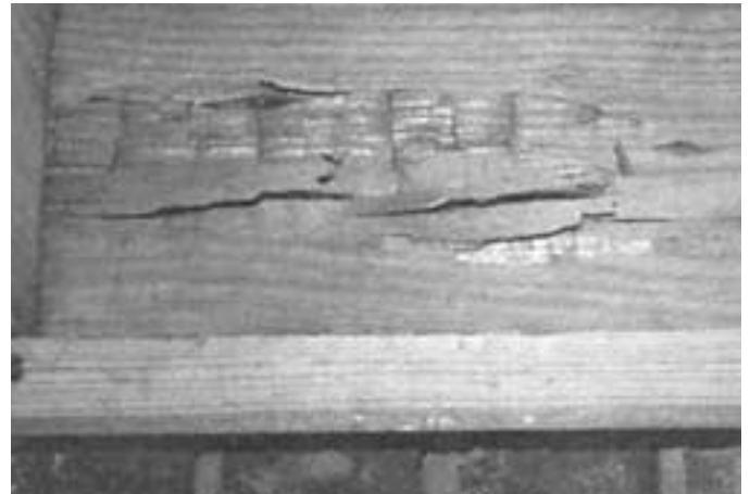
Figure 7.2. Wood damaged by Poria , with apparently sound surface and severe rot below surface.
