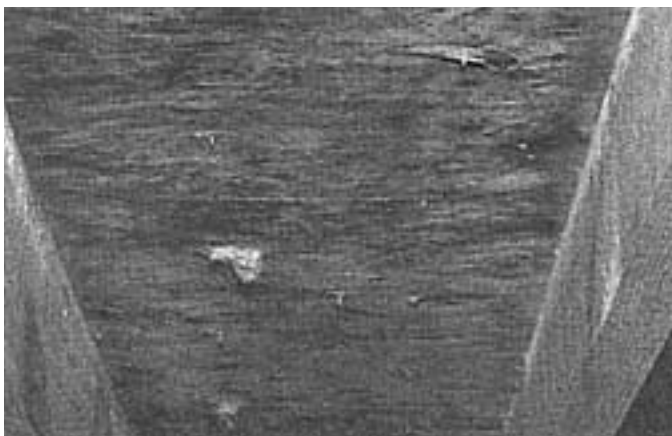
Figure 7.8. Surface molds on plywood attic.
